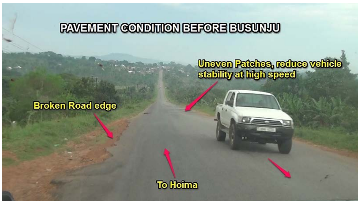
Figure 2: Typical Pavement Condition of Kampala-Busunju Road Section
